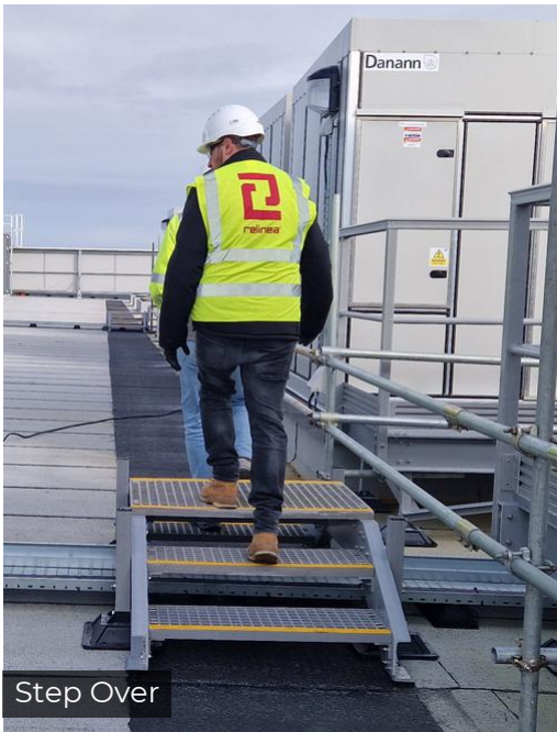
Data Centre Rooftop Access Platforms
